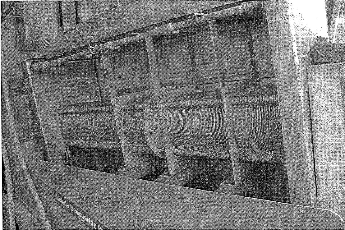
Figure 25: PW Tech Pilot System Photograph during Onsite Pilot Testing
