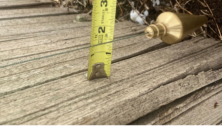
South Shed Walls – 1 1/2" out of Plumb over 5'
