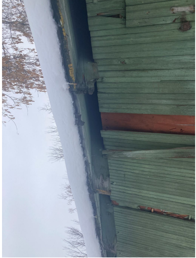
South Shed – Rafter/Siding Condition
