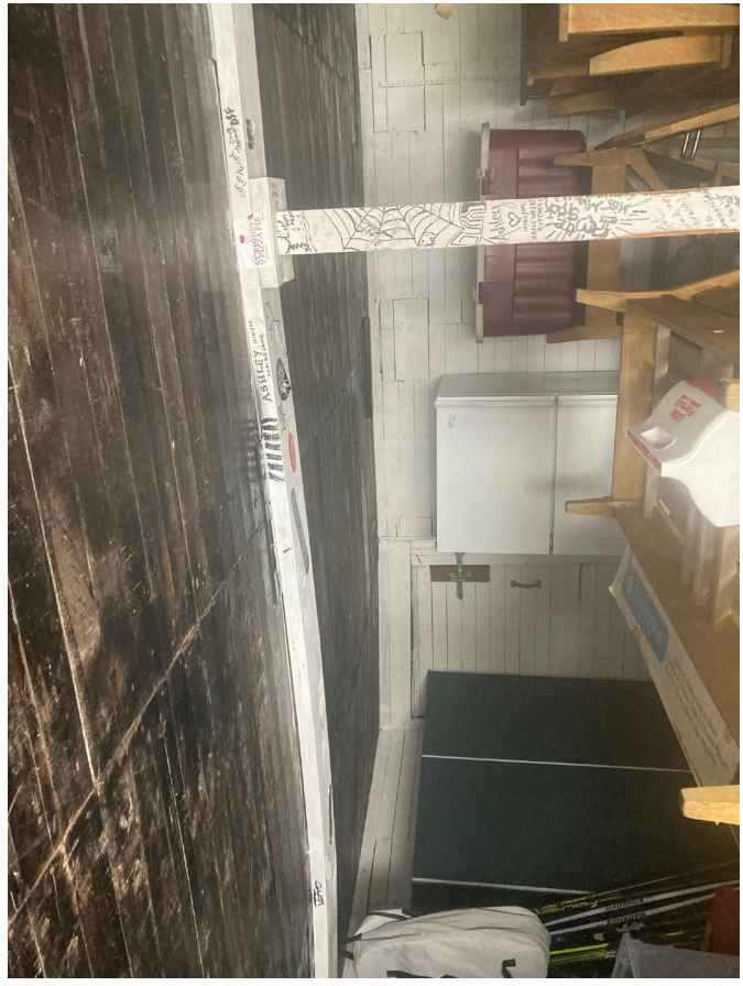
South Shed – Sagging Ceiling and Inadequate Beam
