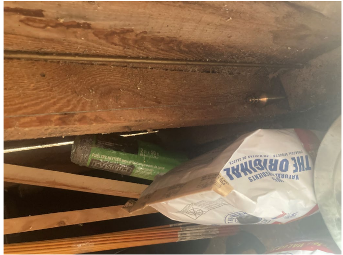
North Shed Wall Studs – 1 1/4" out of Plumb over 6'
