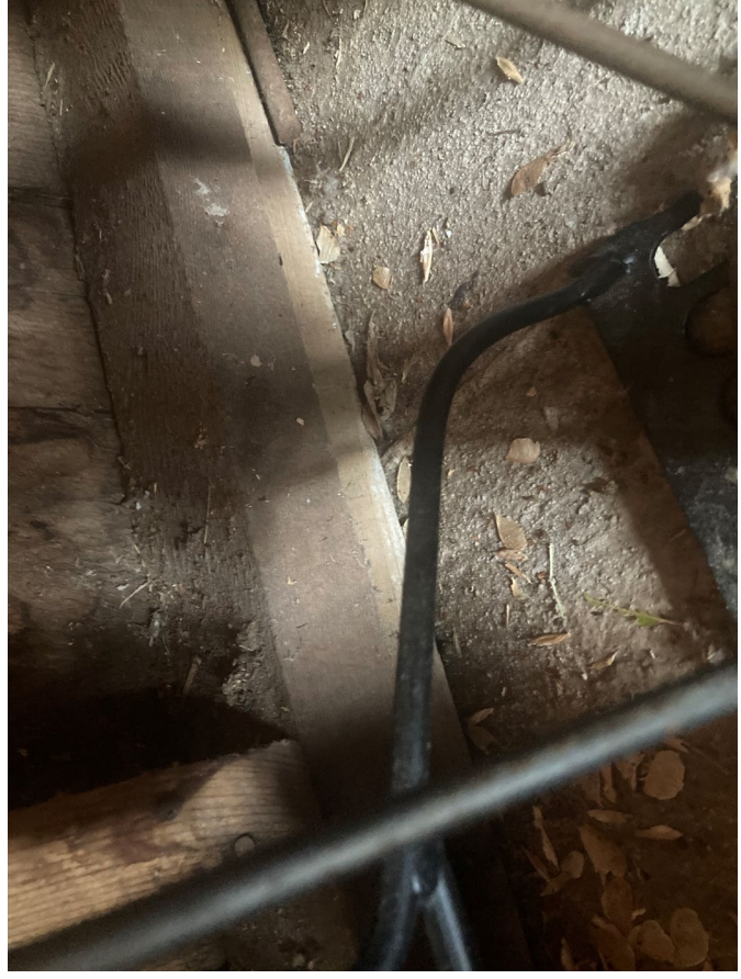
North Shed Sill Plate – no Anchors
