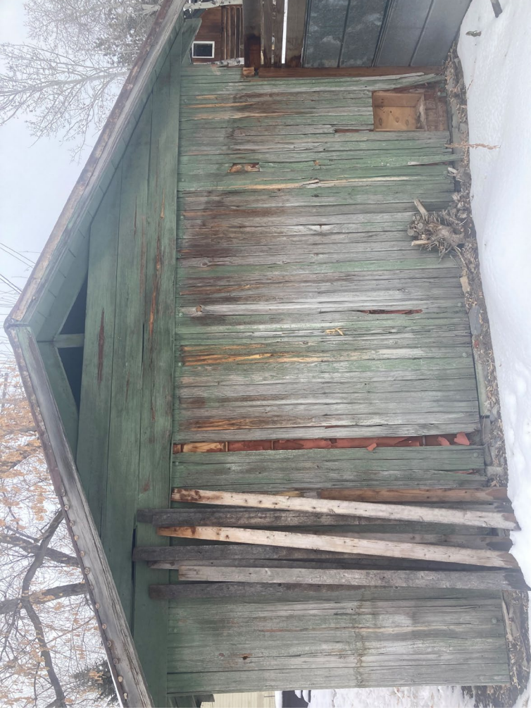
South Shed – Siding Condition, Lack of Foundation
