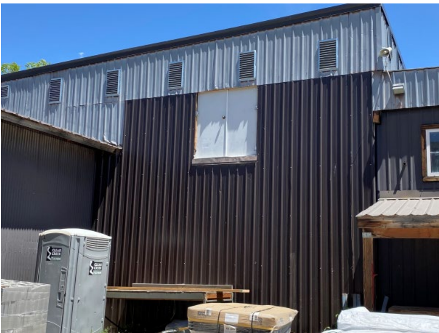
WEST ELEVATION (PARTIAL) – ADDITION TO STORAGE WILL BE IN THIS AREA AND TO THE SOUTH
