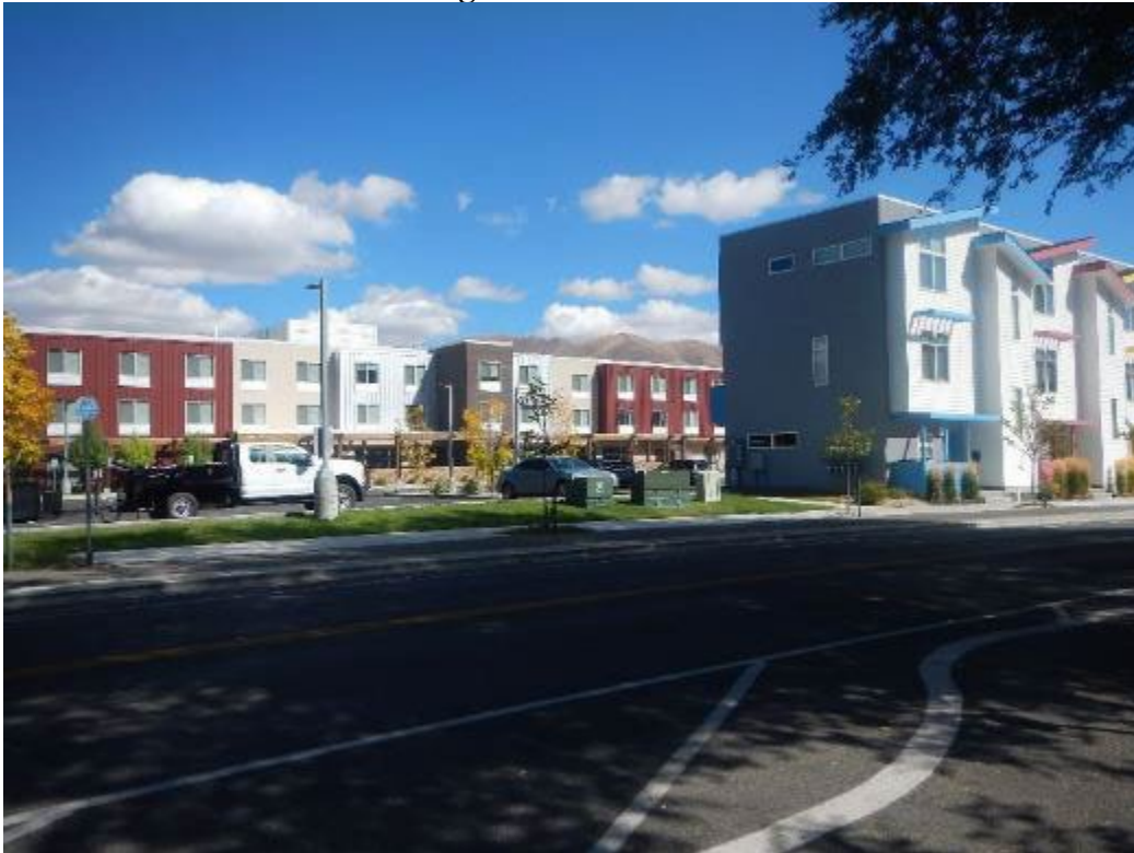
Photo 16: Electrical transformers located on Fairfield Inn property across River Street Note: no leakage of transformer oil observed.
