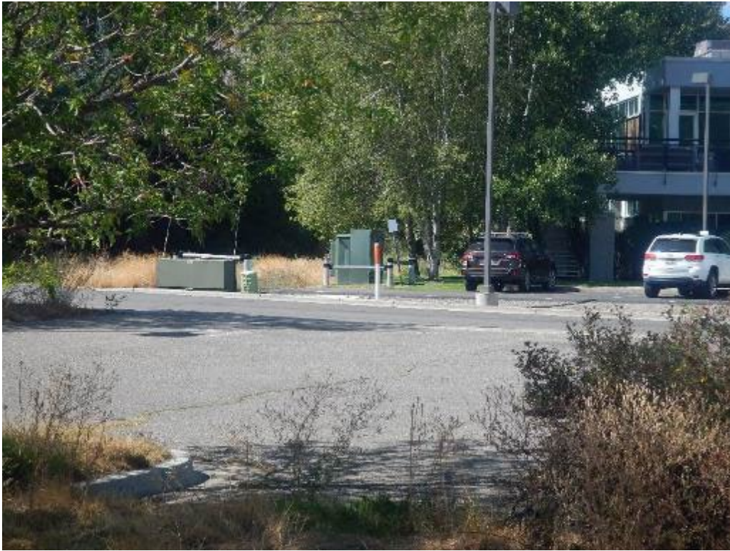
Photo 15: Nearest visible electrical transformers on property across Empty Saddle Trail Note: no leakage of transformer oil observed
