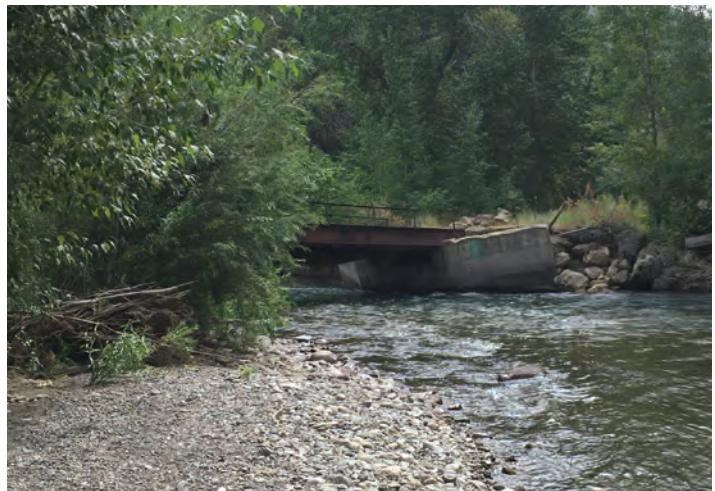
DAMAGED BRIDGE AT COLORADO GULCH TO BE REPLACED
