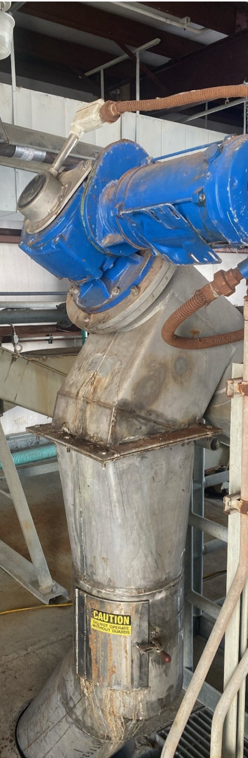
HEADWORKS - WASTEWATER TREATMENT FACILITY
