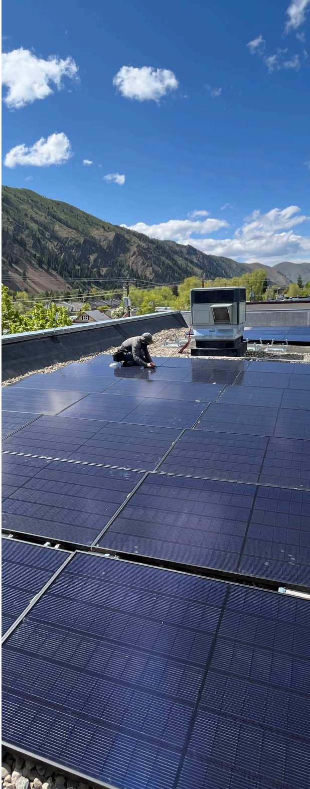
SOLAR INSTALLATION ON THE CITY HALL ROOF
