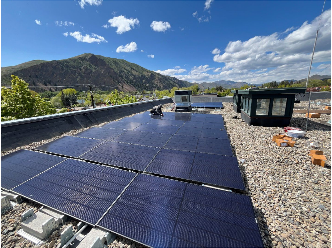
Hailey City Hall Solar Array
